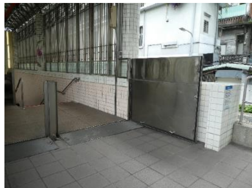
Figure 21. Partial-height flood door at entrance to Taipei Metro (photo: R. Sterling)
