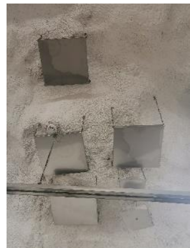
Figure 19. Drip pans in the Helsinki pedestrian tunnel system (photo: R. Ting)
